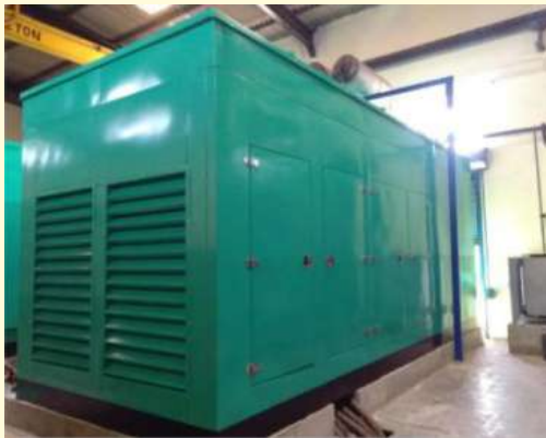
ACOUSTIC CANOPY FOR DIESEL GENERATOR SET IN STEEL PLANT
